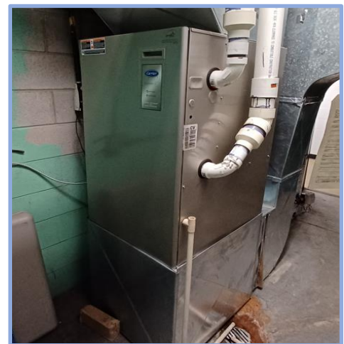
Propane Furnace: Typical of (2)
