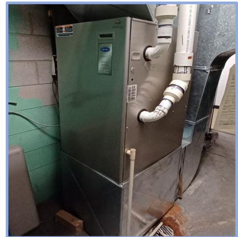
Propane Furnace: Typical of (2)
