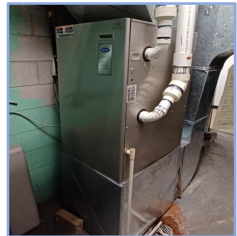
Propane Furnace: Typical of (2)
