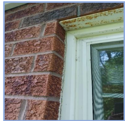
Window Frame: Caulking in Poor condition
