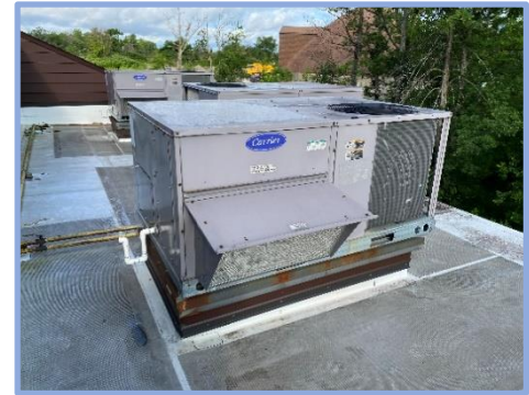
Packaged Rooftop Unit – Typical of (4)
