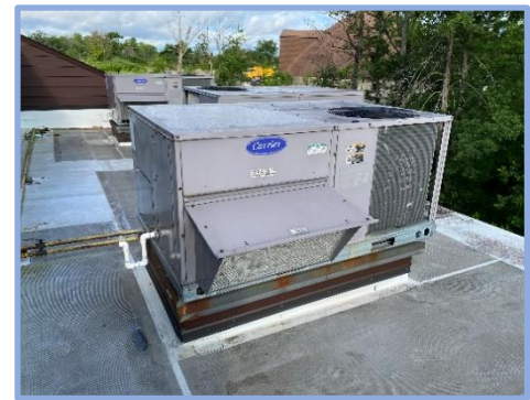
Packaged Rooftop Unit – Typical of (4)
