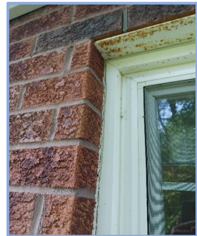
Window Frame: Caulking in Poor condition
