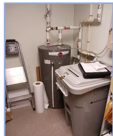
DHW Heater - Electric
