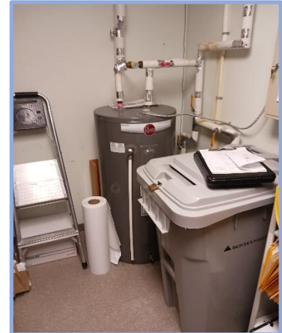
DHW Heater - Electric
