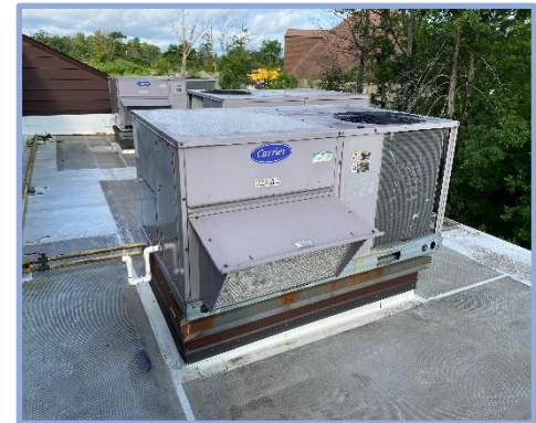
Packaged Rooftop Unit – Typical of (4)
