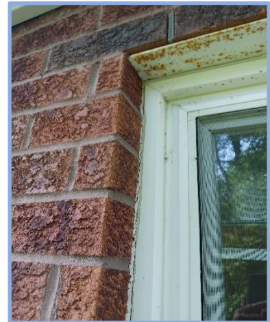
Window Frame: Caulking is Cracked and Degraded
