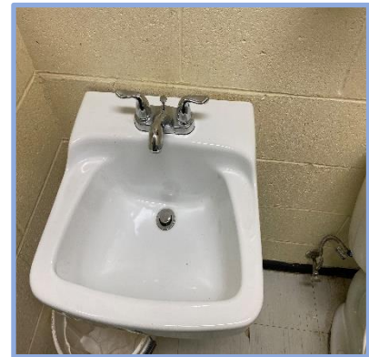
Faucet in washrooms
