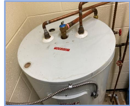
Domestic Hot Water Tank
