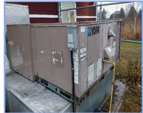
Ground Mounted RTU
