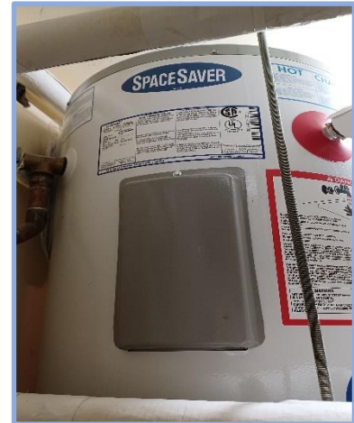
Domestic Hot Water Tank
