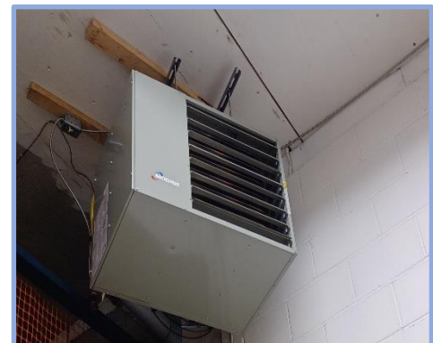
Propane Unit Heater
