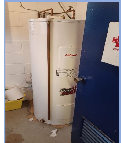
Domestic Hot Water Heater Tank
